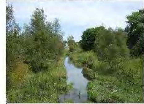
20090828 Terry Fox Culvert sediment & vegetation build-up since 1972
