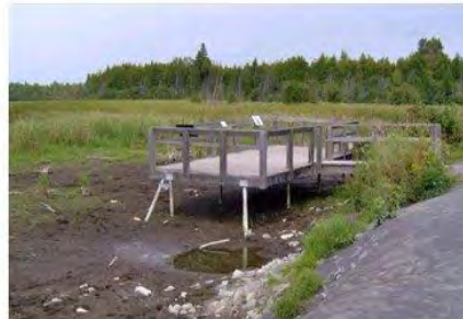
2 Sep 2011 Upper Poole Creek Wetlands after beaver dam removal and culvert replacement
