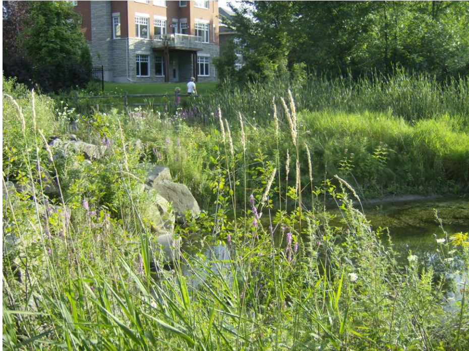
This is taken from the Beaver Pond side of the rock wall and shows the forebay outlet culvert which allows the stormwater to flow to the Beaver Pond
