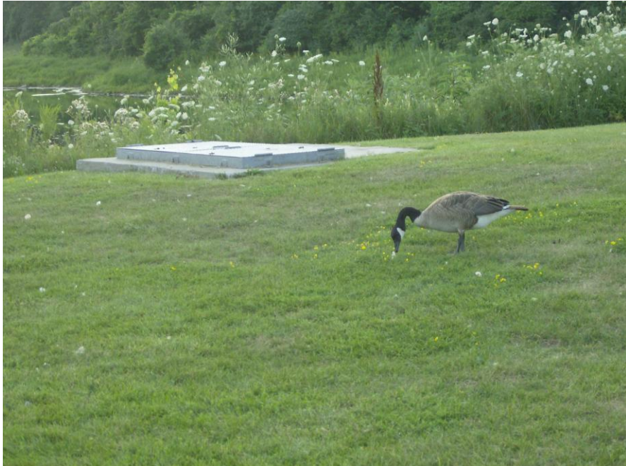
This access structure is at the top of the east-end path. There is a shallow grassed swale aligned with this towards the parking lot, which may be due to settling of the earth when the culvert was installed.
