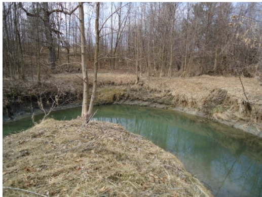
Figure 5: Erosion of the Banks
