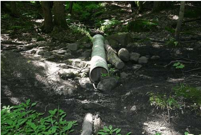
Figure 31: faulty culverting and expanded impact area along mountain bike trail
